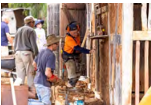
Learning how to in-fill a timber frame wall at Rechner Cottage, Light Pass pugging workshop, 2024, Sam Kroepsch
